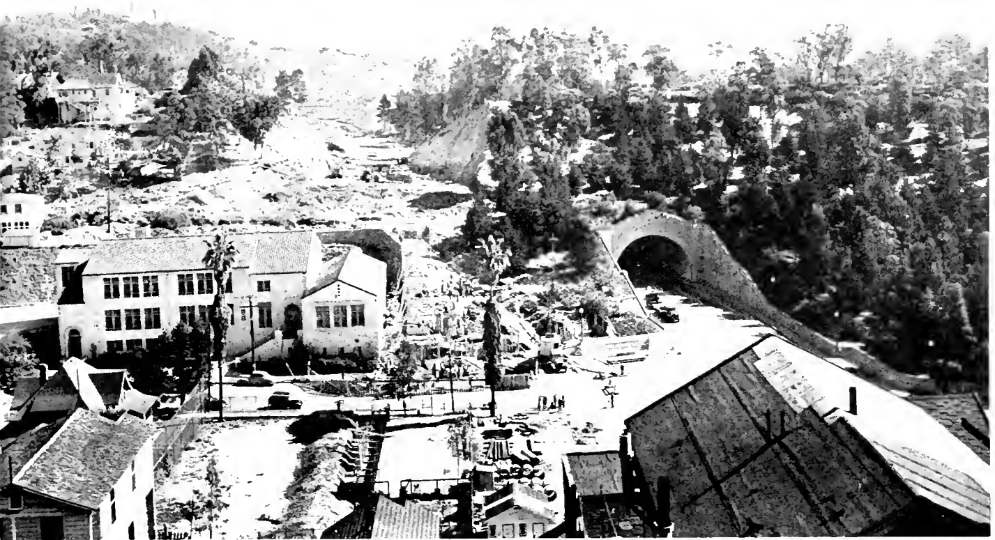
View of open cut under construction through Elysian Park in Los Angeles for southbound traffic extension of Arroyo Seco Freeway
